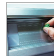
Drill Holes at the marked location & insert wall plugs in the holes.
